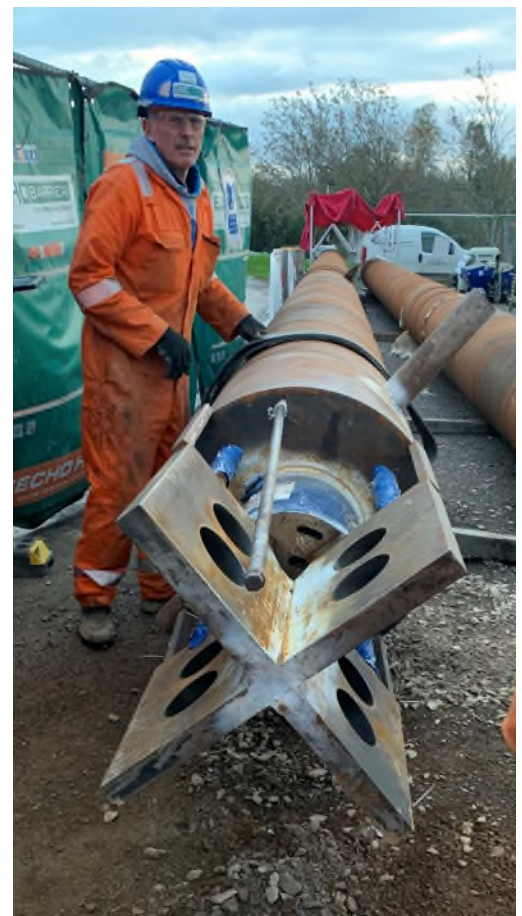
O-Cell® assembly on the bottom of the steel pipe pile ready for installation
