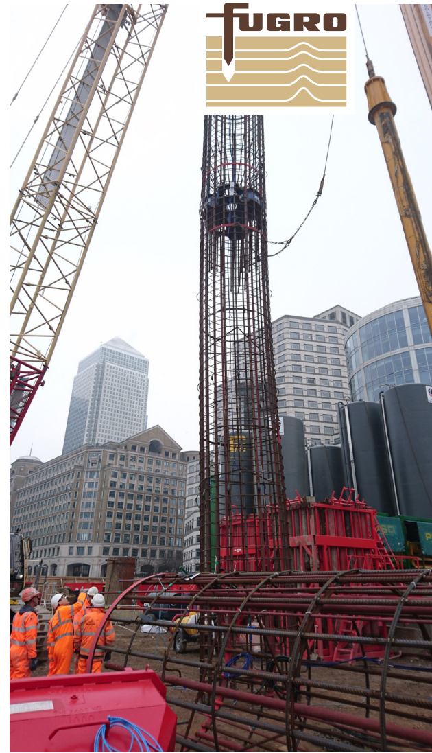
Installation of the reinforcement with three 670 mm O-cells for the first test pile.
