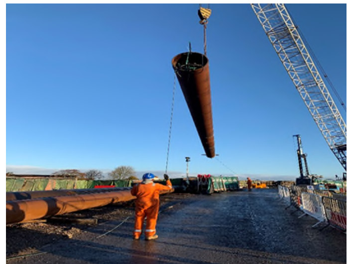
Pipe pile and O-Cell® assembly ready for installation into the bore and grouting
