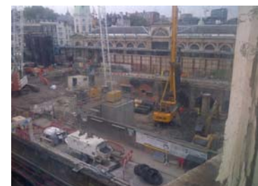
O-cell testing made the perfect solution on the congested sites at Crossrail
