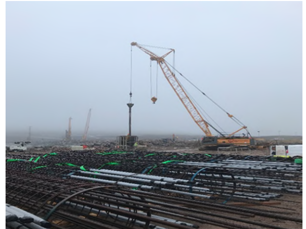
Installation of the reinforcing cage and instrumentation ready for into the pile
